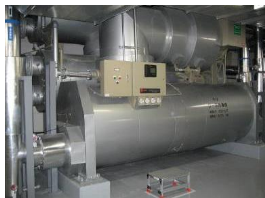
High-efficiency turbo refrigerators
