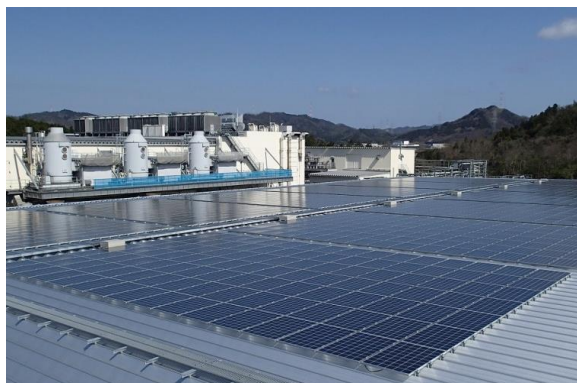
Solar power generation system on the rooftop of the Kyoto Ayabe Plant (1.6 MW)
